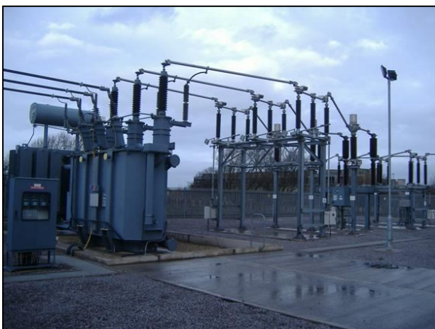
Photograph 5 132kV Grid Substation: main power conductors at high level
