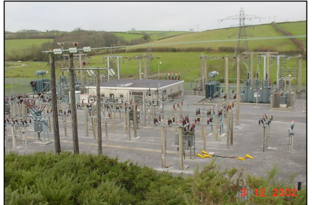
Photograph 2 132kV Grid Substation
