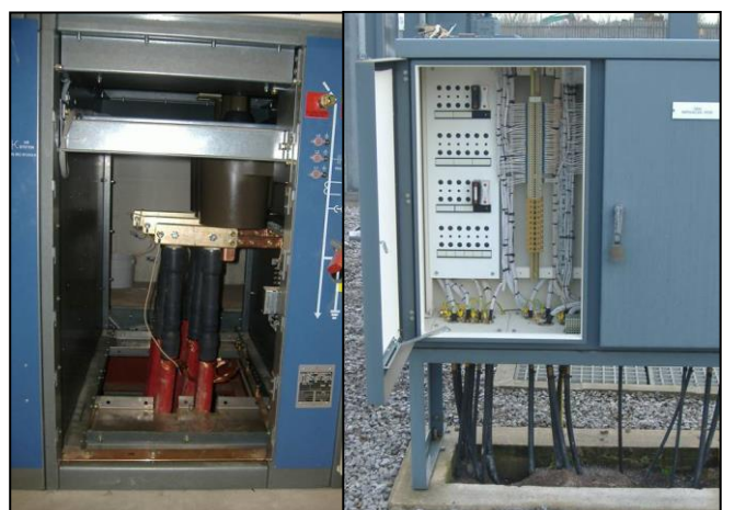
Photograph 6 Primary Substation: low-level conductor in HV switchgear & control wiri
