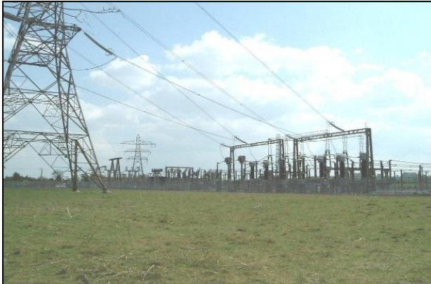
Photograph 1 400kV Transmission Substation
